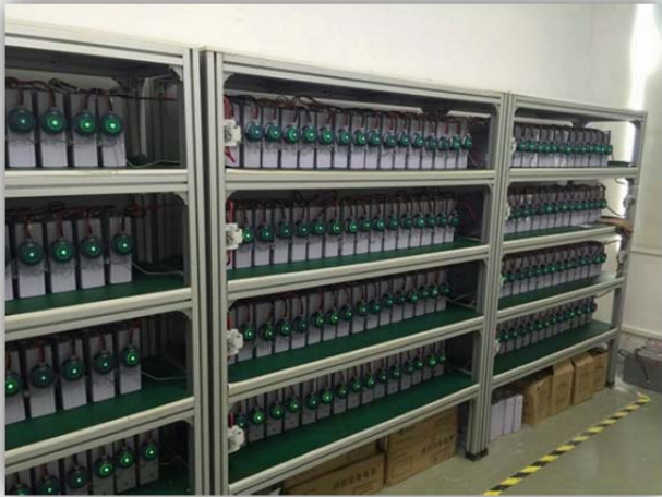
FIGURE 2 BATTERIES WITH SENSORS IN BATTERY BANKS
